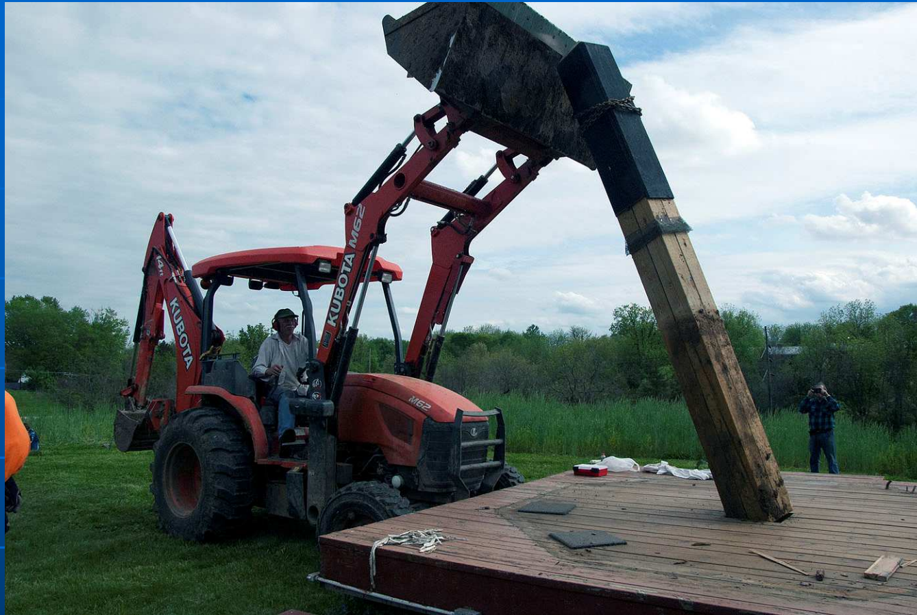
Mr. Nordick used his tracker lift and pulled the telescope post out of the ground, which was buried in five feet.
